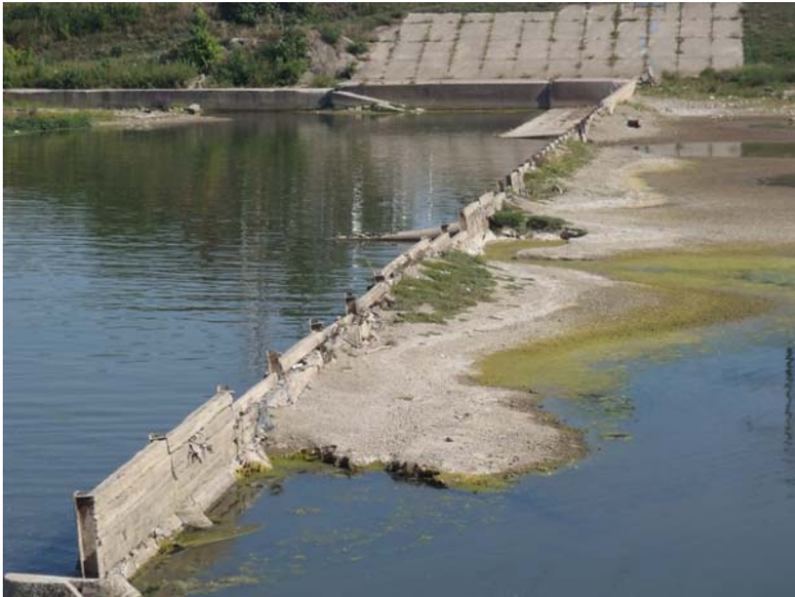
Time Lapse Removal of a Low Head Dam on the Great Miami
